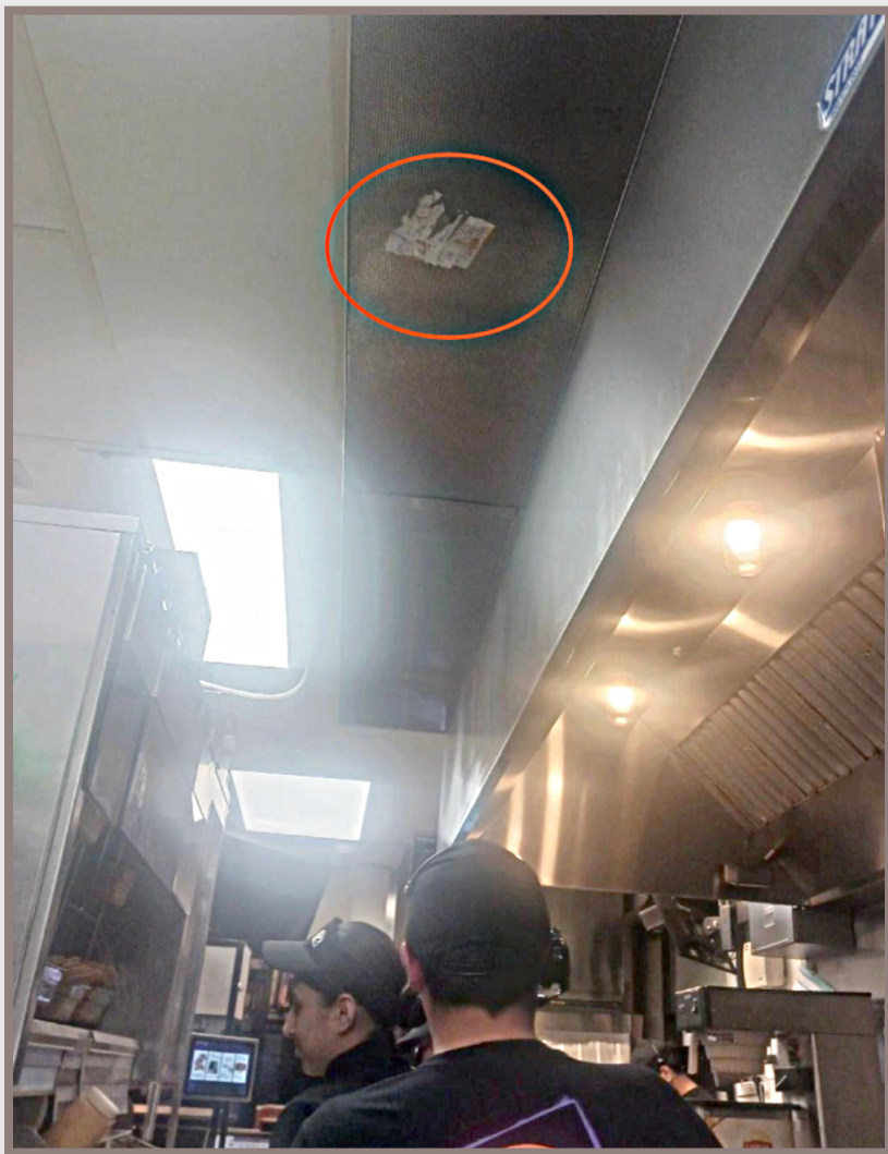
9/6/2024: Workers at a Taco Bell in Culver City placed stickers on ceiling tiles to try to block rain water from leaking through the roof above the food prep line.
