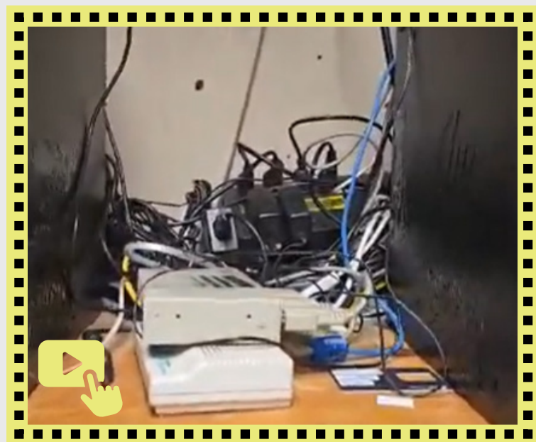
Image from video of rain dripping through ceiling onto electronics, potentially causing electrocution and fire hazards.
